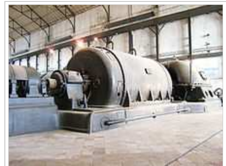
Early Ganz Generator in Zwevegem, West Flanders, Belgium
