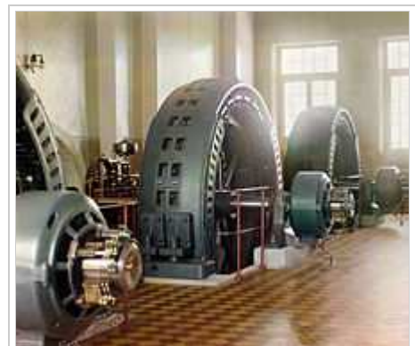
Early 20th century alternator made in Budapest, Hungary, in the power generating hall of a hydroelectric station
